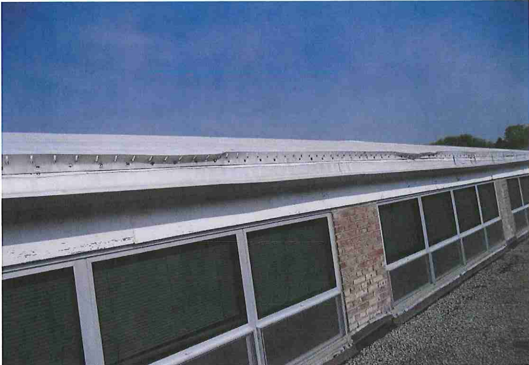
Old 1991 roof system showing failures
