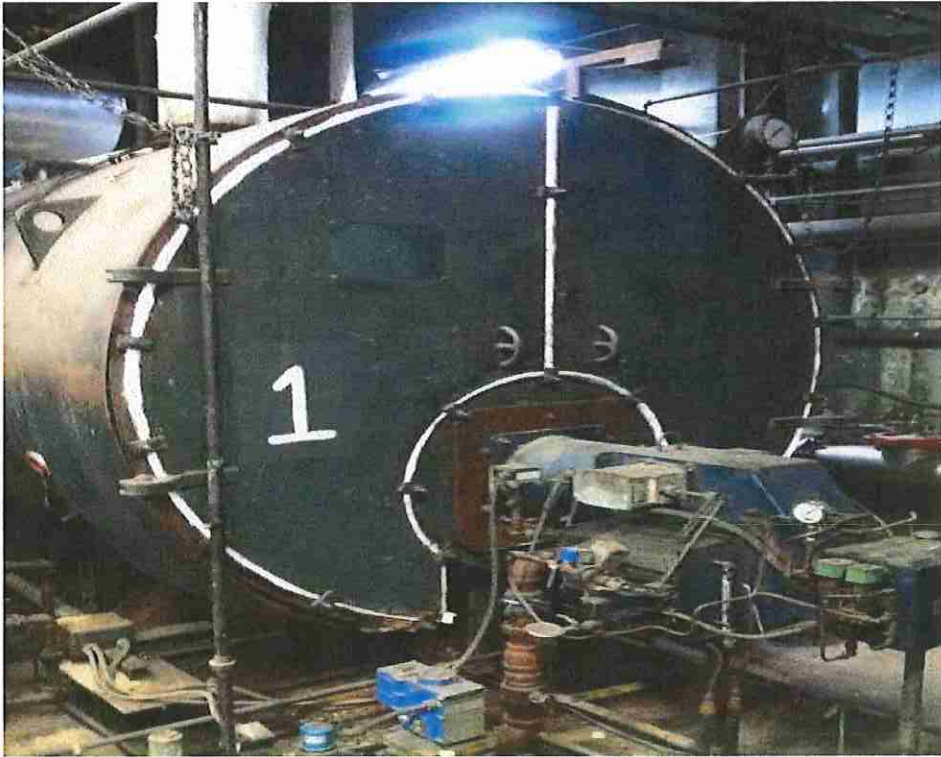
Old 1971 boiler #1 showing age and fractured wall section
