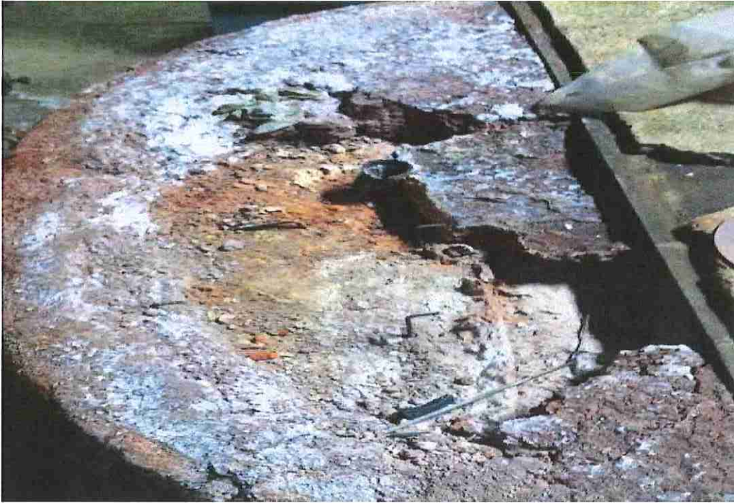
Close up of fractured sections
