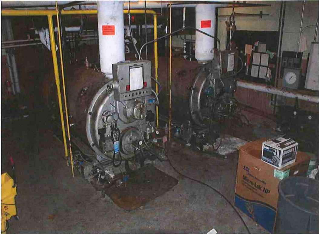
Old 1964 boilers showing age and leaks
