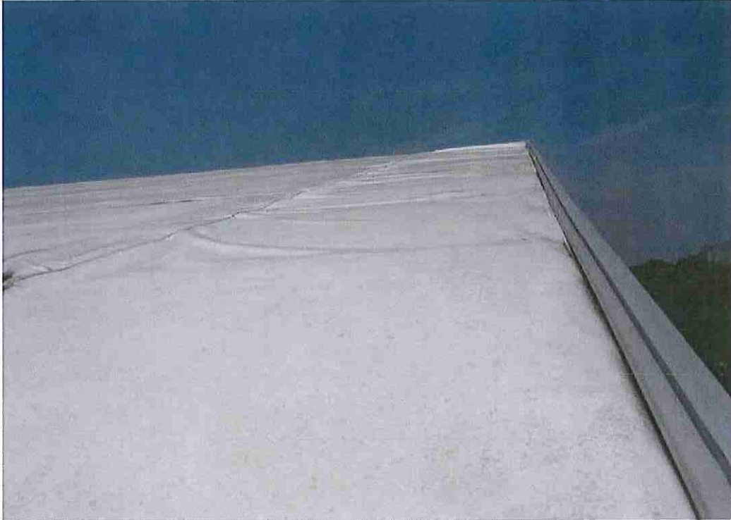
Roof membrane failures and patches around skylight
